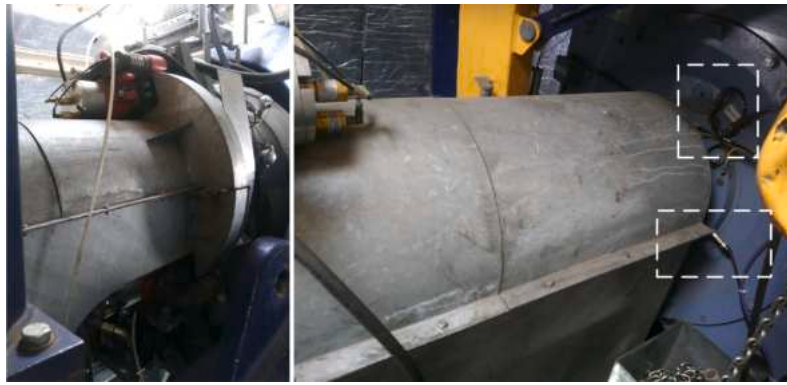
Fig. 3. Installation locations of vibration accelerometers on the wind turbine generator, mounted horizontally and vertically (Chen et al., 2021).
